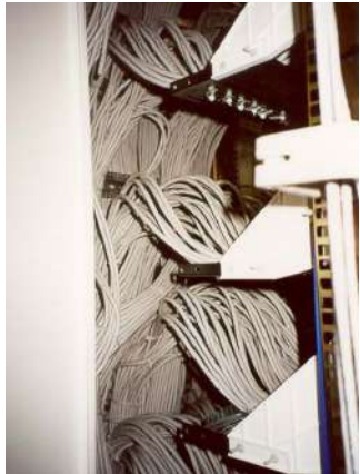
Wrong rack cable management, to big bundles
